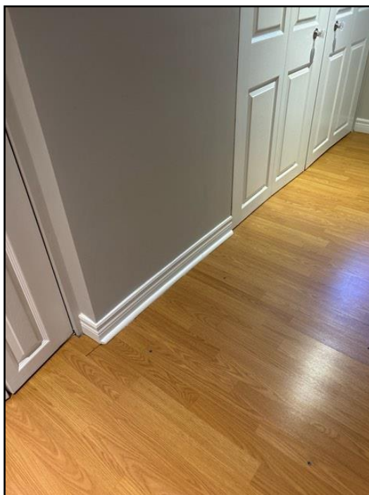
Backwater valve not visible
