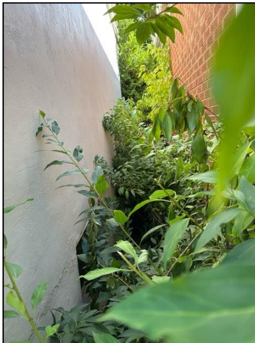
shrubs too close to building
