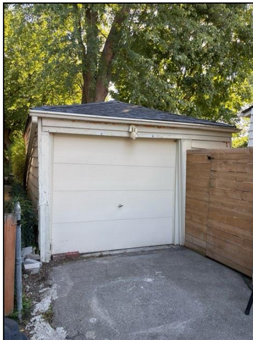
Typical low quality structure
