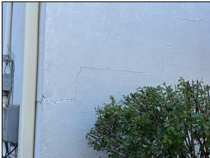
Masonry - small cracks...
