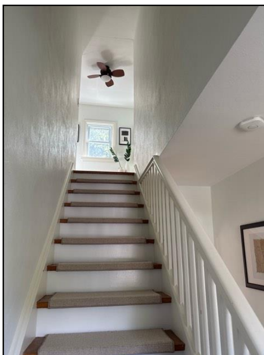
Incomplete or not continuous railing
