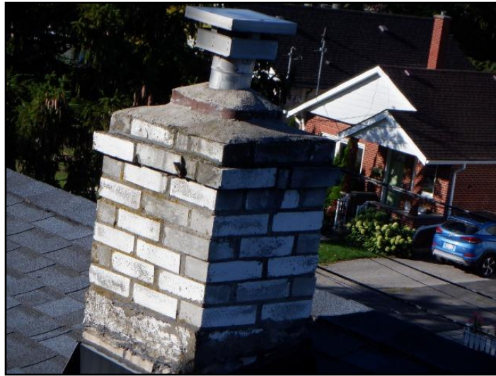
Missing masonry chimney cap
