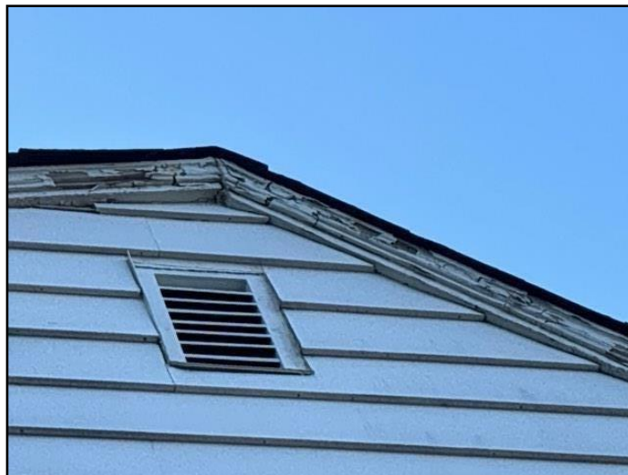
Paint or stain - deteriorated / missing
