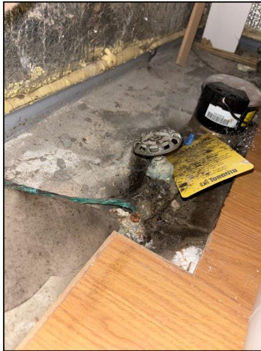
Difficult to access
