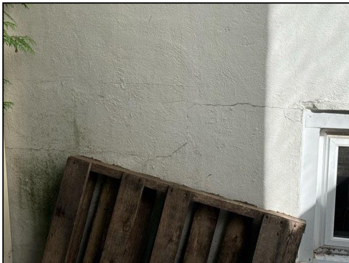
Masonry - small cracks...
