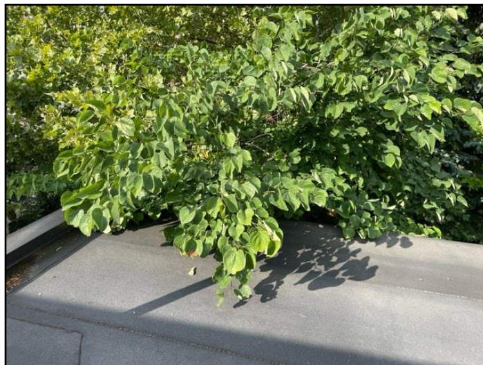
Tree branches touching roof
