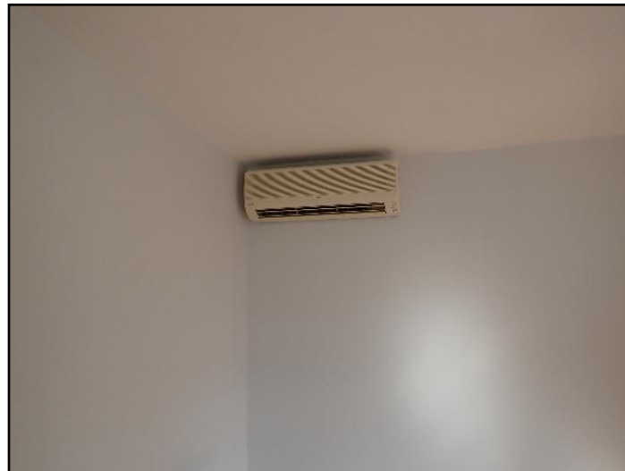
Indoor unit - Second floor front - Fujitsu
