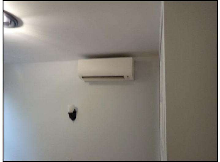
Indoor unit - Second floor rear - Daikin
