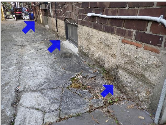
Unsealed gap at building
