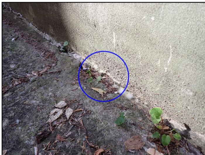
Unsealed gap at building
