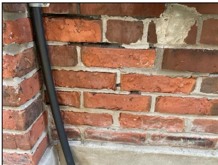
Spalling brick - Right side front
