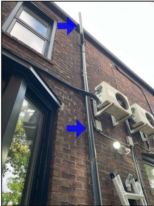
Waste vent stack
