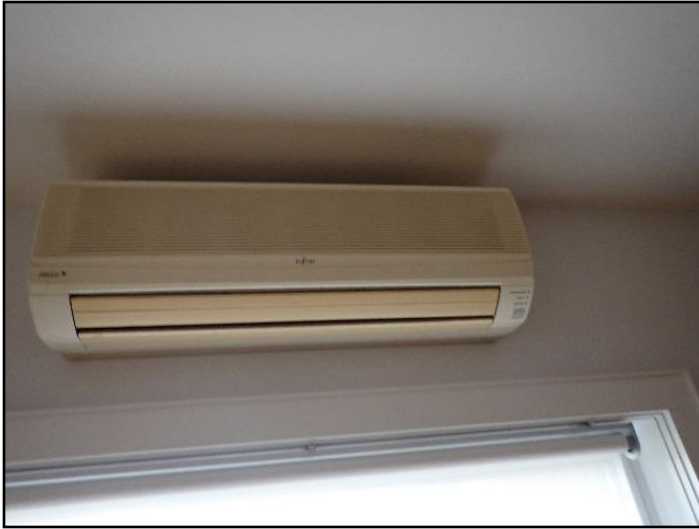
Main floor Indoor unit - Fujitsu
